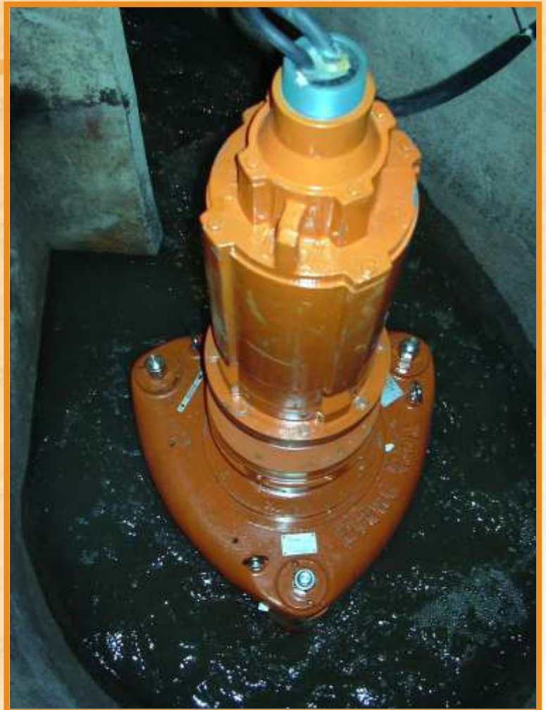
Basin of previously installed Chicago Pump 25M
