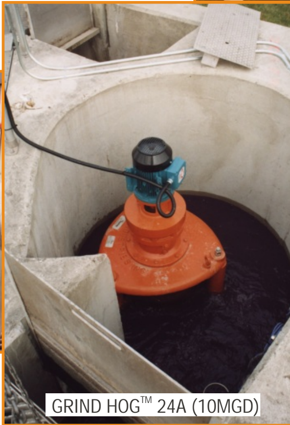
PREVIOUSLY INSTALLED CHICAGO 25A
